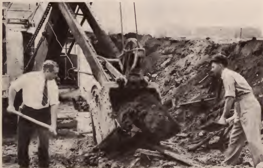
Apparently dissatisfied with the work that lusty steamshovel is doing in excavating for WGY's new building, William T. Meenam, Press Relations, and Willard J. Purcell, engineer, took shovels in hand and helped out a bit. A wide-awake cameraman caught them tucking in shovelfuls of dirt into corners of the shovel. Things are coming right along, incidentally, with the new building. Of course, the noise outside the present studios hasn't reached the rat-a-tat riveting stage yet, but the chug-chug sound of the shovels continues.
