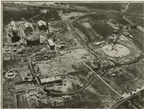
Aeroplane view of the new Mineral Springs Road Plant of the Iroquois Gas Corporation.
