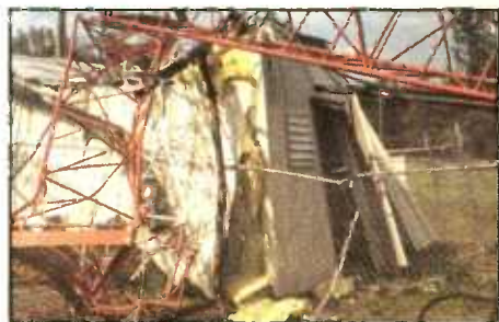
Opal's power had devastating effects on radio towers in Columbus, Ga.
