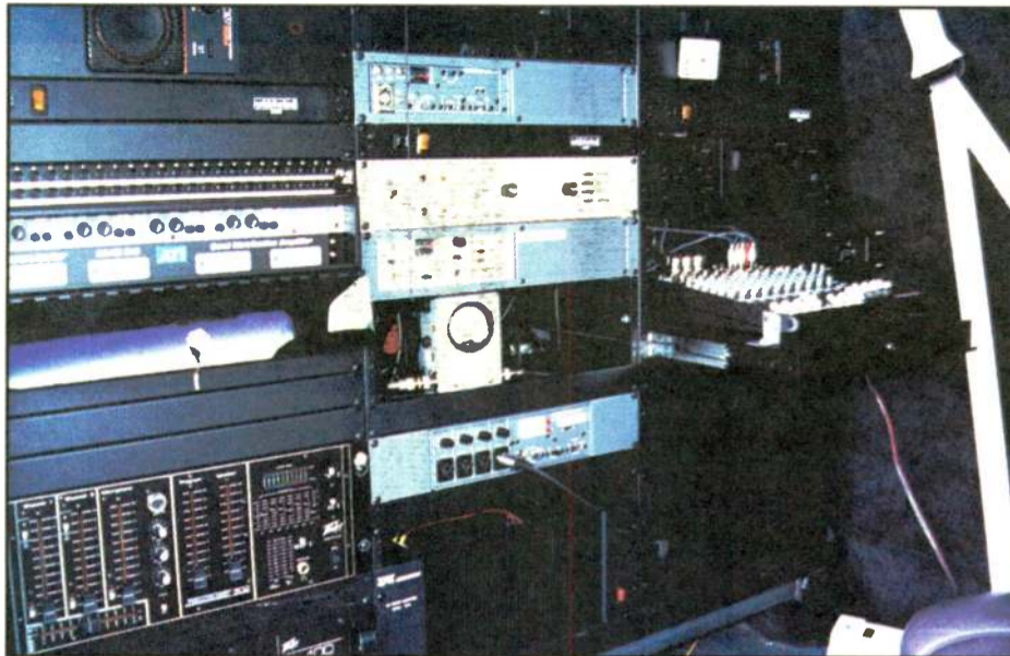
The WQBQ van has three equipment racks installed across its width.
