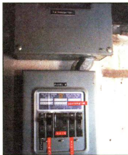
Figure 2: Labeling circuit breakers takes a short time, and the payoff can be life-saving in an emergency.
