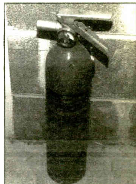
Figure 2: Keep a fire extinguisher by the door to your transmitter building ... and make sure it's charged!
