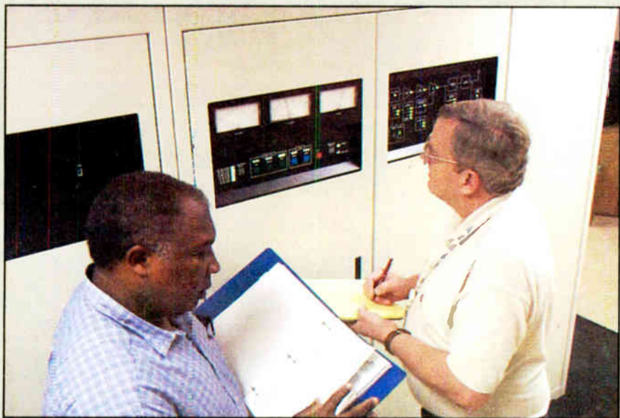
Senior engineer David Jones (left) and Walt Taylor, a WSB engineer, work at the DX 50.
