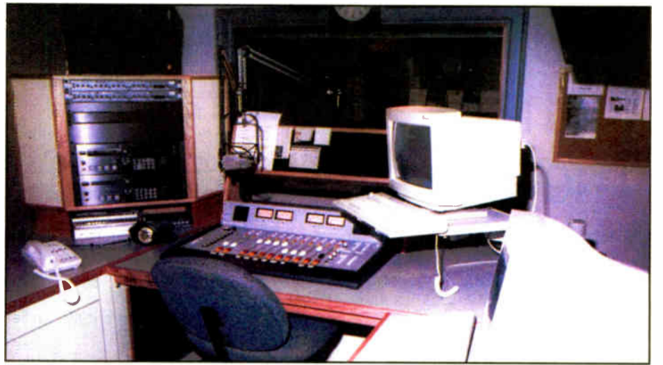
The new on-air studio at Radio Voyager is built inside former WGAY office space. A Scott Studios DOS-driven automation system runs the show during unattended hours.
