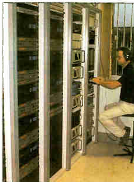
An NTL employee operates the multi-plex for commercial radio in the U.K.
