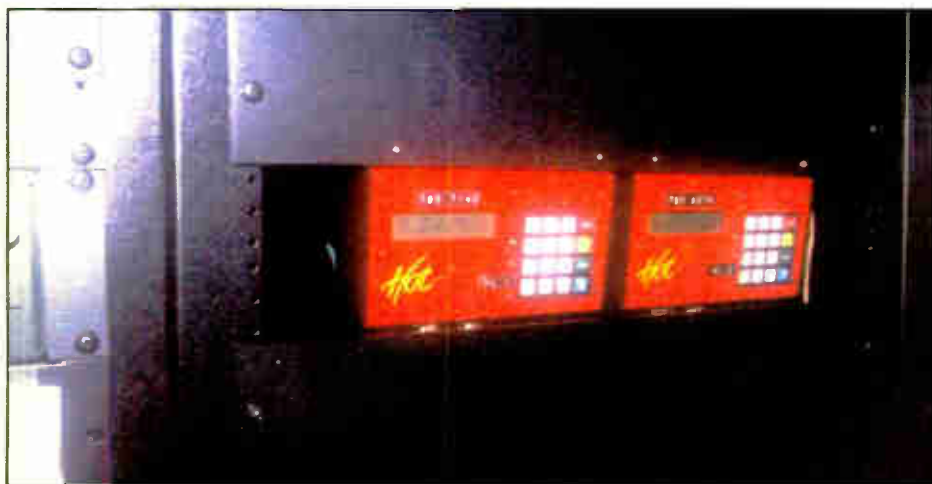
Figure 1: Here's an inexpensive equipment mount, using blank rack panels.
