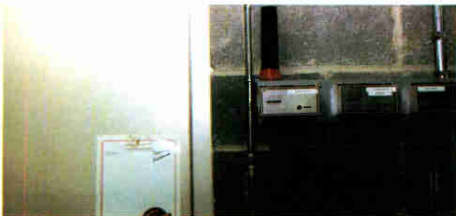
Figure 2: Can you find four things done right at this transmitter site?
