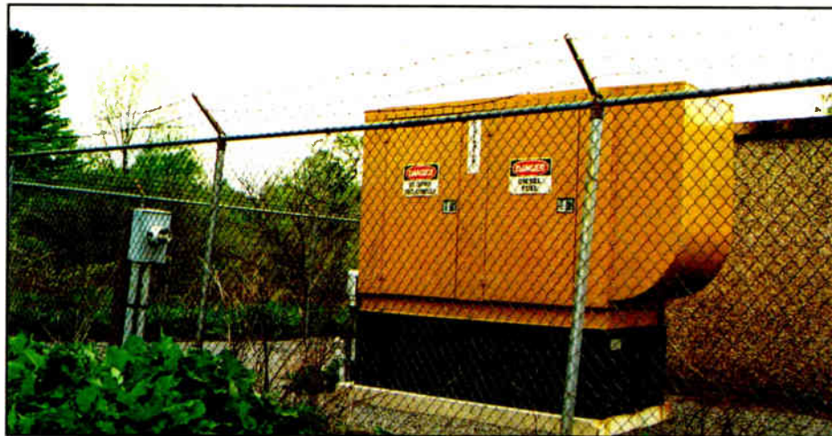
Signs and fences can save lives and fend off tremendous liabilities. The signs read 'Danger: This Equipment Starts Automatically' and 'Danger: Diesel Fuel.'
