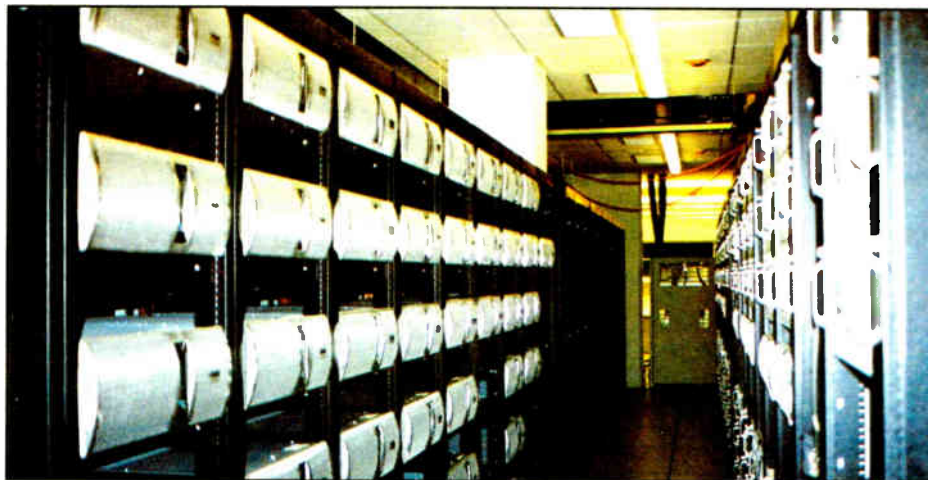
XM's Technical Operating Center
