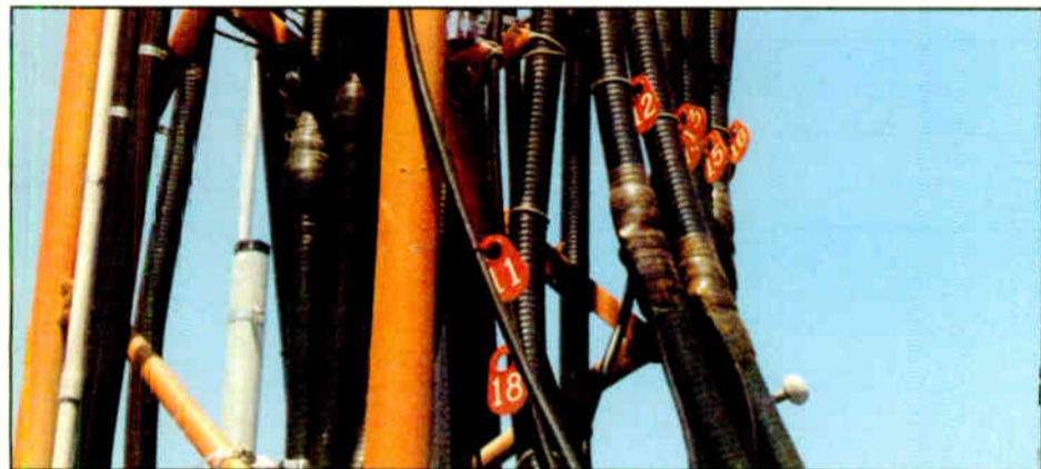
Fig. 1: Check the security of grounds on your transmission lines
