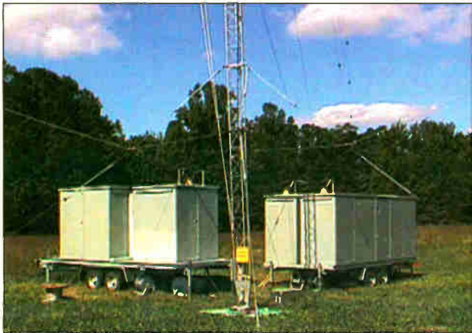
Photo 2: Mobile triplexer installed at tower base
