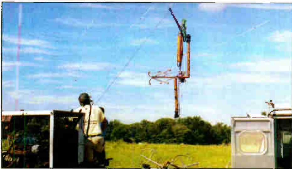
Antenna installation for WMMO(FM)
