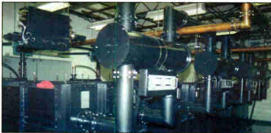
The Dielectric combiner system at American Towers, Blitho tower in Blitho, Fla.
