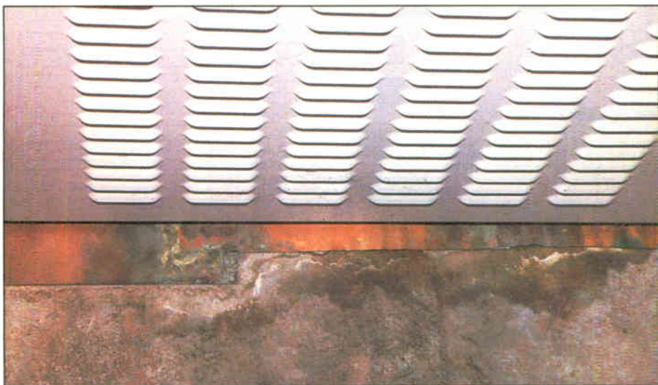
Fig. 1: Water leaks can damage equipment
