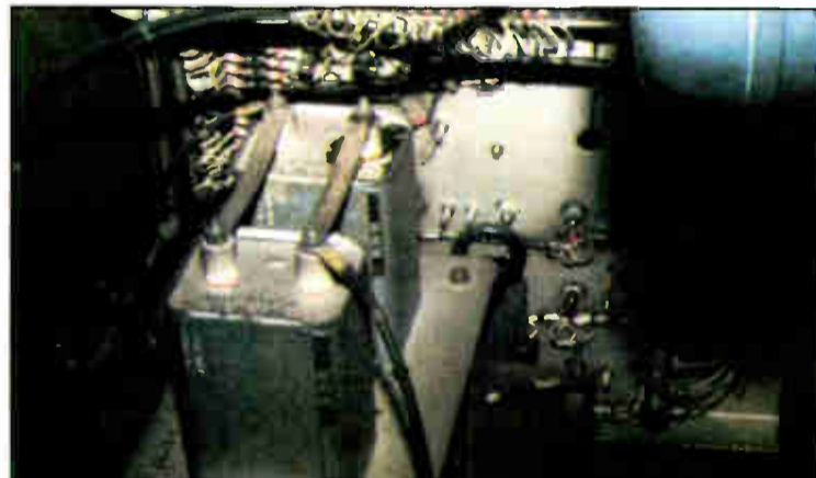
Fig. 2: Bring along a strong trouble light to inspect components inside dark equipment cabinets.
