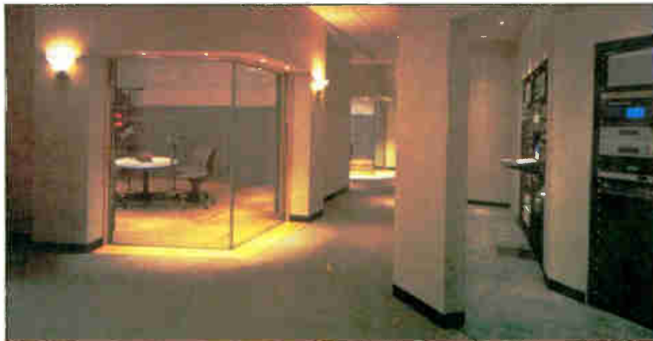
The wire management systems incorporated into the architectural design at Nashville Public Radio (WPLN) eliminate some time-honored traditions: exposed cable trays and wires strung across the floor.
