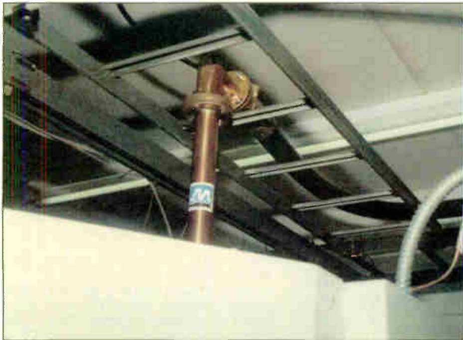
Fig. 1: This cable tray supports the line until it exits the building.
