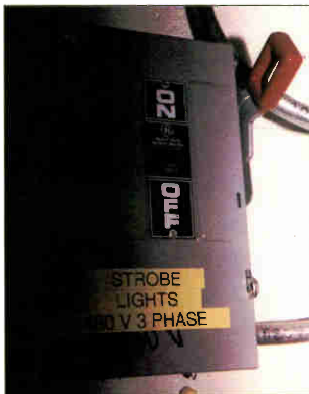
Fig. 7: Use a labeling machine to identify disconnects and other important locations.
