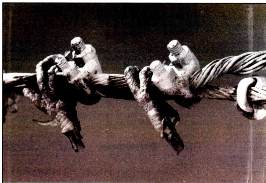
Fig. 3: This is an unpleasant reminder that we work with lethal voltages in radio.
