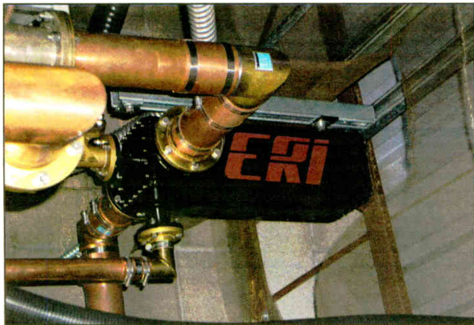
The analog and digital signals feed an ERI 10 dB combiner on the way to the ERI antenna.
