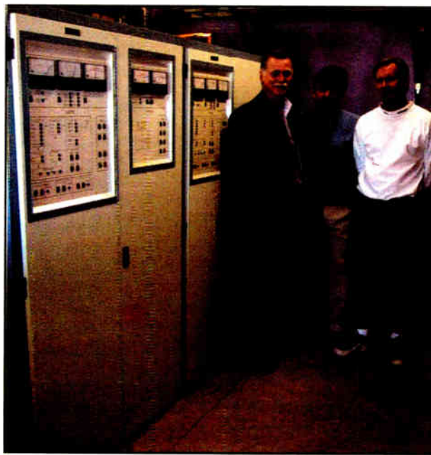
Lotus Broadcasting Director of Engineering Lindy Williams, left, Arizona Lotus Assistant Engineer Dave Shelton and Chief Engineer Gregg Garcia, far right, stand in front of KCMT's new Nautel 40kW solid-state FM transmitter.
