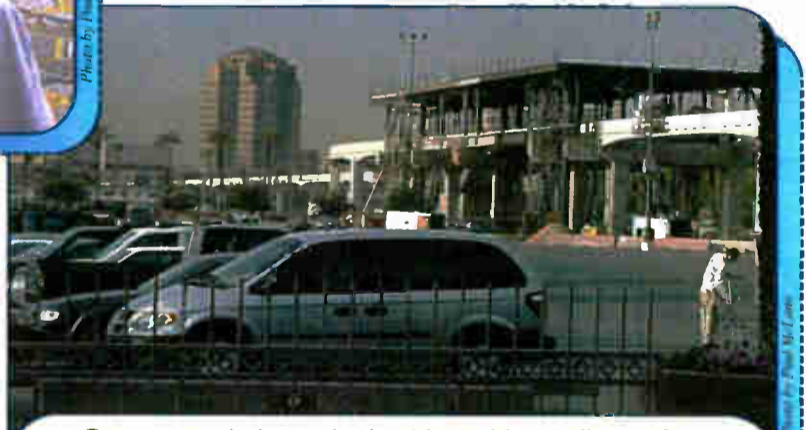
By next year's show, the Las Vegas Monorail, running along the east side of the Strip and stopping at seven stations including the LVCC, will make it easier to move around the city. The LVCC station is shown under construction.
