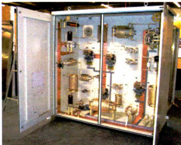
DIRECTIONAL ARRAY ANTENNA TUNING UNIT GAITHERSBURG, MD
