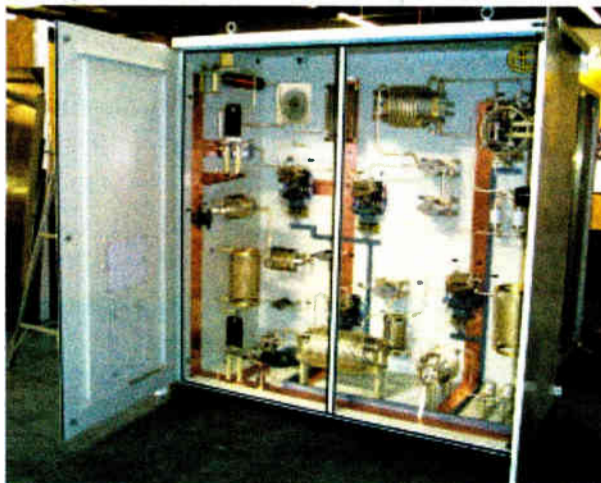
DIRECTIONAL ARRAY ANTENNA TUNING UNIT GAITHERSBURG, MD
