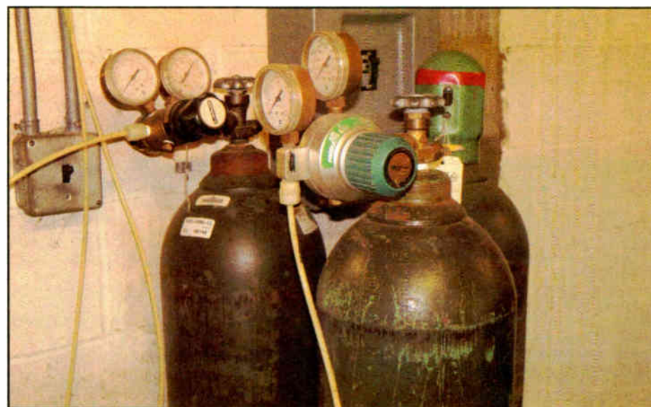
Fig. 3: Check your nitrogen tanks or dehydrators regularly; if the system is leaking, get it fixed.
