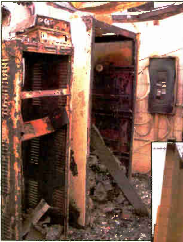
The interior of the KSGN transmitter building after the fires.
