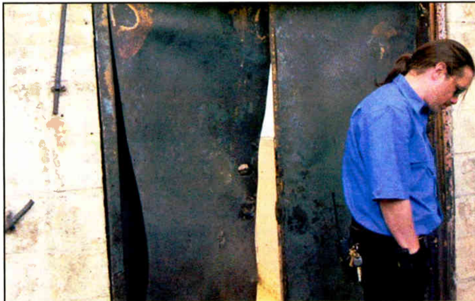
KFRG Chief Engineer Kevin Scott inspects fire damage at the transmitter site.
