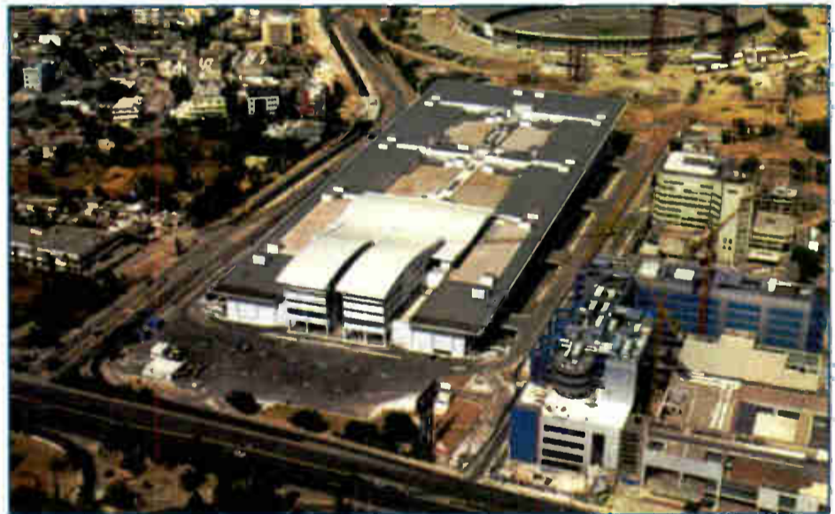
The International Broadcast Center and Main Press Center are shown under construction last fall.
