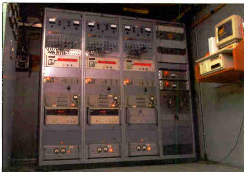
Control room for WWV, broadcasting time and frequency information. This screened room contains electronics to generate the time and frequency signals and voice announcements.
