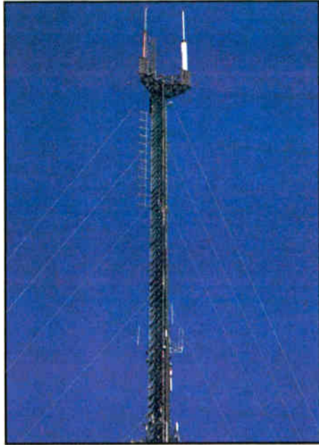
A Dielectric 12-bay DCR-M antenna serves WJCT(FM) in Jacksonville, Fla., sharing space with WJCT(TV)'s NTSC and DTV antennas on a Dielectric tower.
