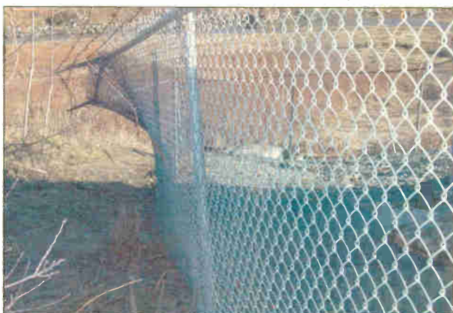
Avoid the fine; repair damaged tower fencing quickly.
