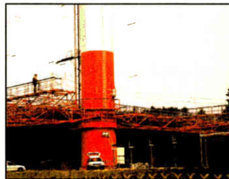
Fig. 5: Wire-Array Tower Base Section
