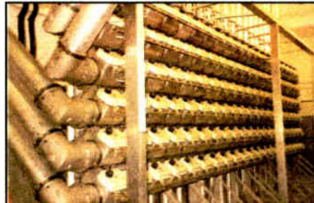
Fig. 2: Coax 6x20 Antenna Switching Matrix at RFE/RL, Maxoquierra, Portugal
