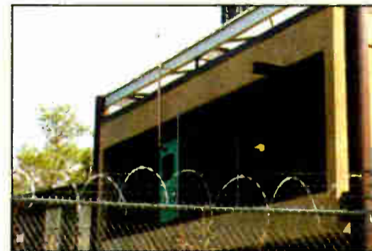
A security fence surrounds Cox Radio's WKHK(FM) in Richmond, Va., where Jon Bennett is chief. A generator is visible on the platform.
