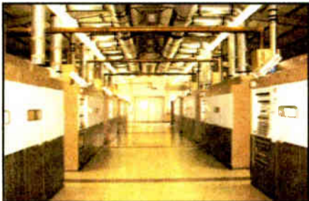
Fig. 1: Typical Transmitter Hall, RFE/RL Biblis, Germany
