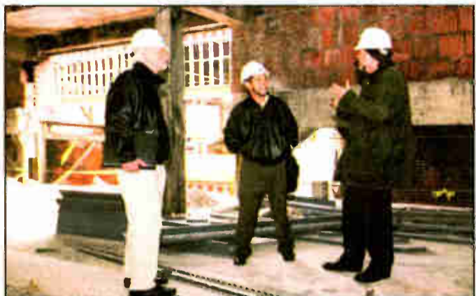
Greg Walters, Hal Real and Roger LaMay survey the project during construction. Real is president of Real Entertainment, LaMay is general manager of WXPN.
