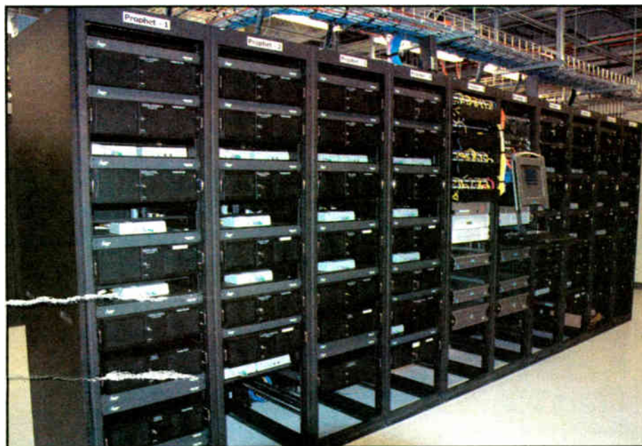
Rack room at Clear Channel's new consolidated facility in Los Angeles. Terry Grieger is chief engineer.
