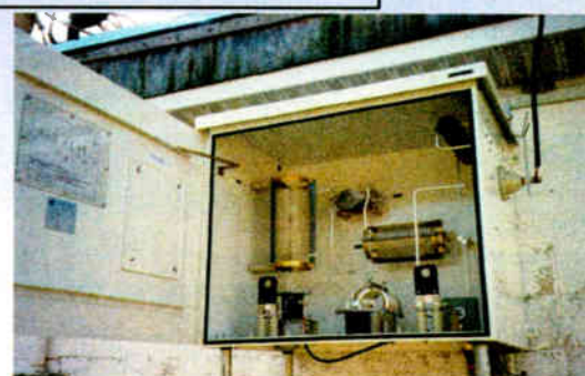
Kintronic Model LTU-1B, 1kW ATU Installed At KSTL-AM/ Crawford Broadcasting—St. Louis
