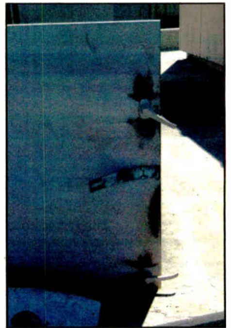
Fig. 3: When half of a 20 MW load is disrupted, it's quite a light show.
