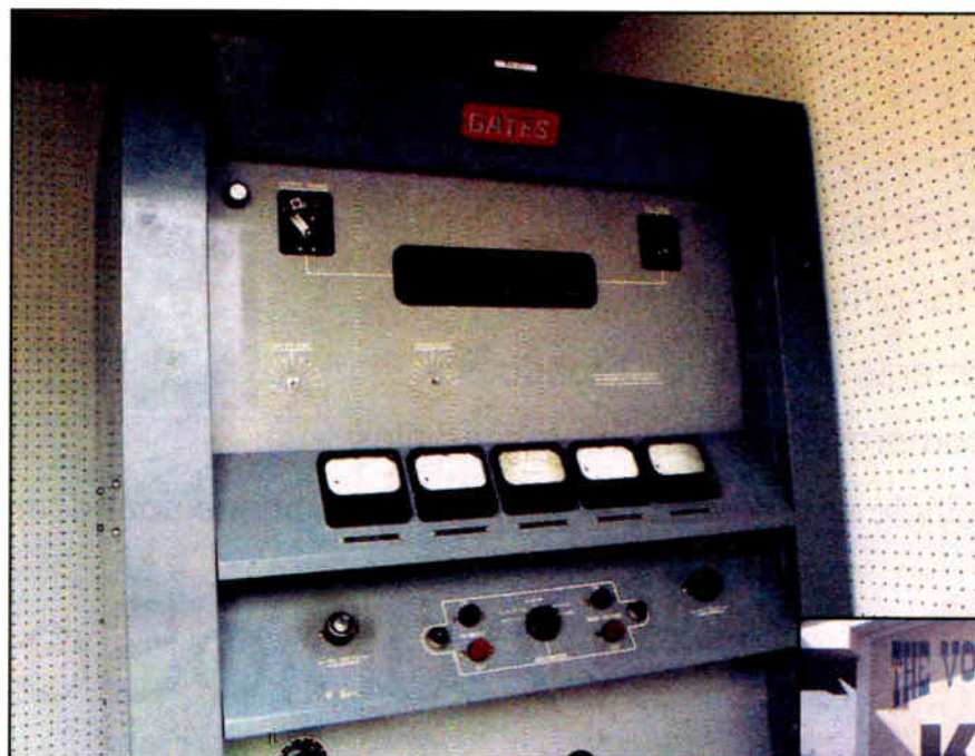
The Gates BC250L transmitter at home in its new pad.
