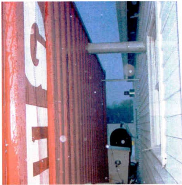
Fig. 2: Conduit is used to link storage containers.
