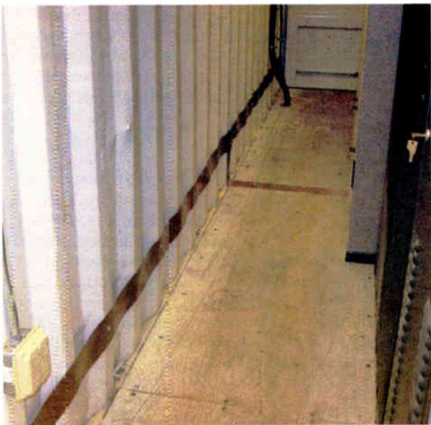
Fig. 1: A nice clean interior for a transmitter shack.
