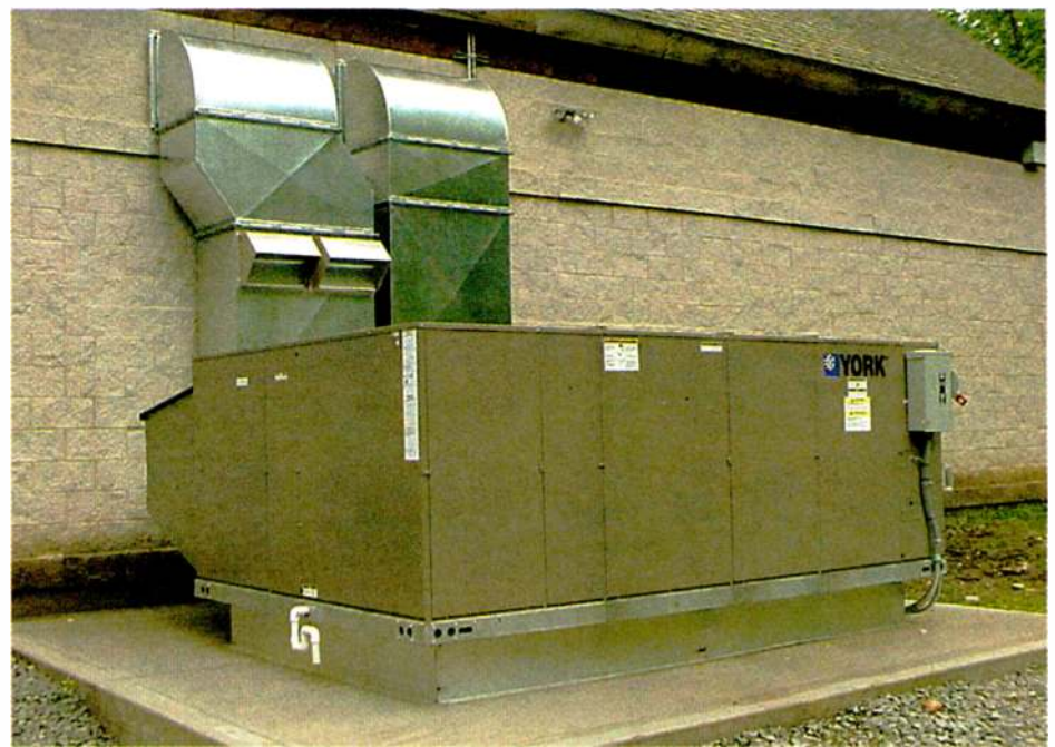
A pad-mounted HVAC system is shown. Note make-up air ducts on left.
