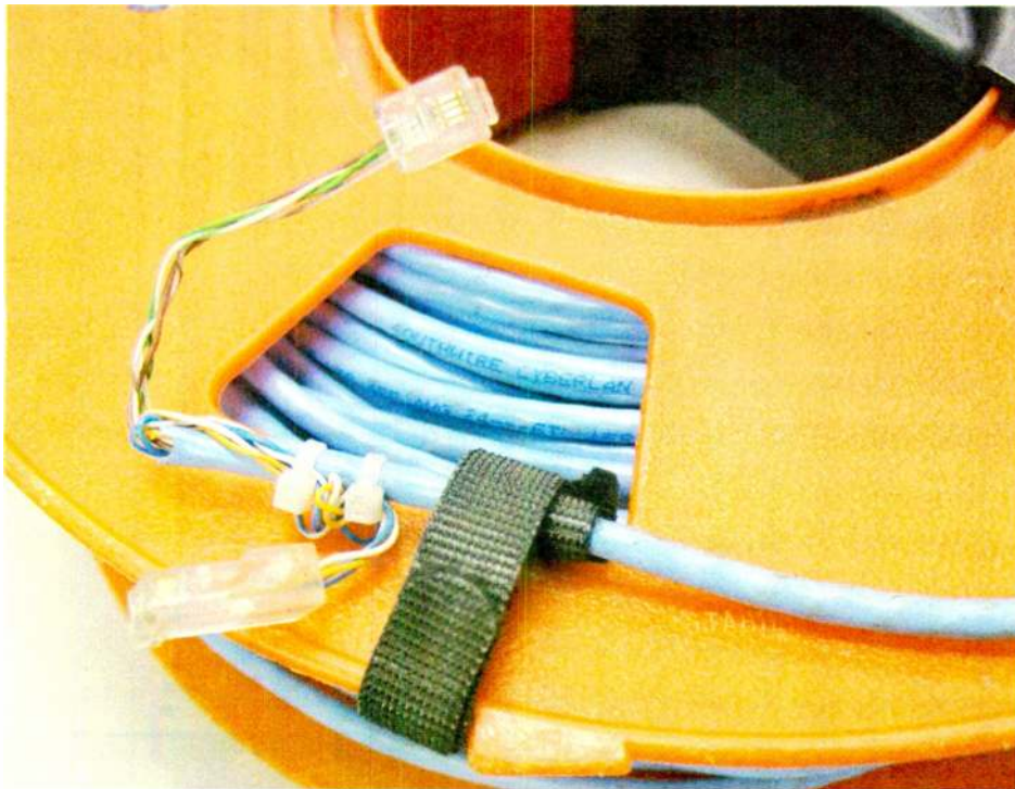
Fig. 3: Velcro brand or other reusable 'hook and loop' straps keep cables secure.
