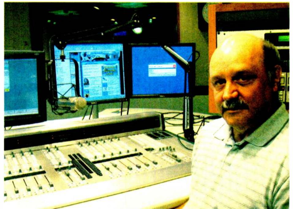
Dave Garner of Bonneville Broadcasting, Washington D.C., seated at one of several Harris consoles in the multistation facility. Pictured here is a Harris RMXdigital console in a production/backup on-air studio for WTWP and WGMS.
