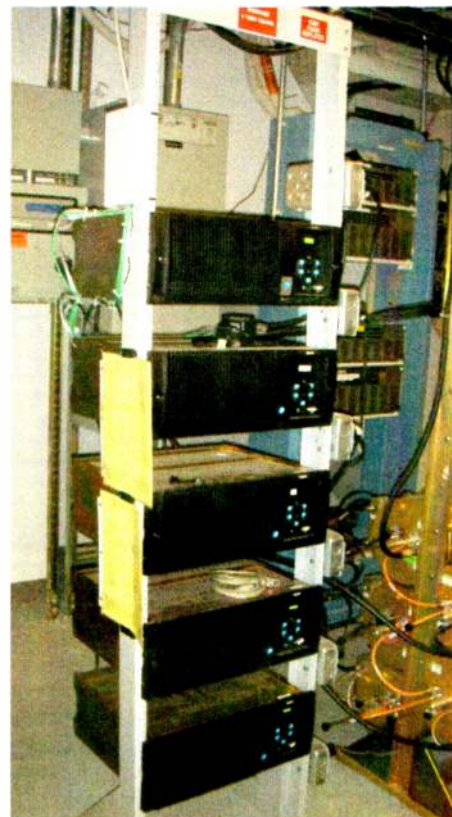
Typical FDNY and Durst Repeater Rack
