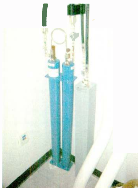
Blue units are Shively 2912 transmitter isolation cavities, gray is the EMR receive bandpass.
