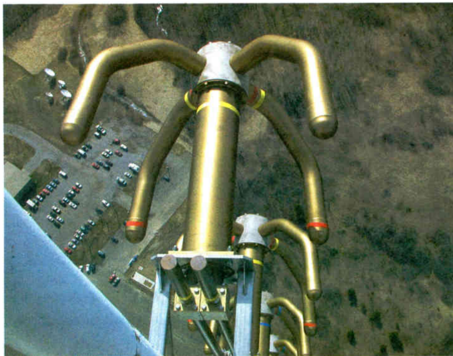
A photo of WRIF's DI-6A antenna bay showing dual feed lines.
