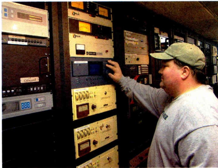
Chris Tarr is Entercom director of engineering for the Milwaukee and Madison, Wis., clusters. Here he tweaks an Optimod 8200, testing the audio processing on the HD2 service of WMMM in Madison.
