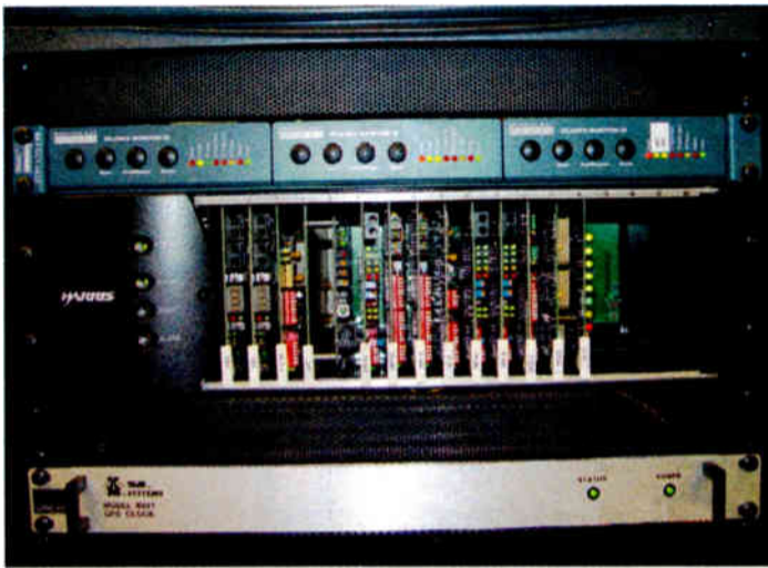
A Harris Intraplex STL system, open, showing a series of modules for T1 distribution, including SynchroCast.
