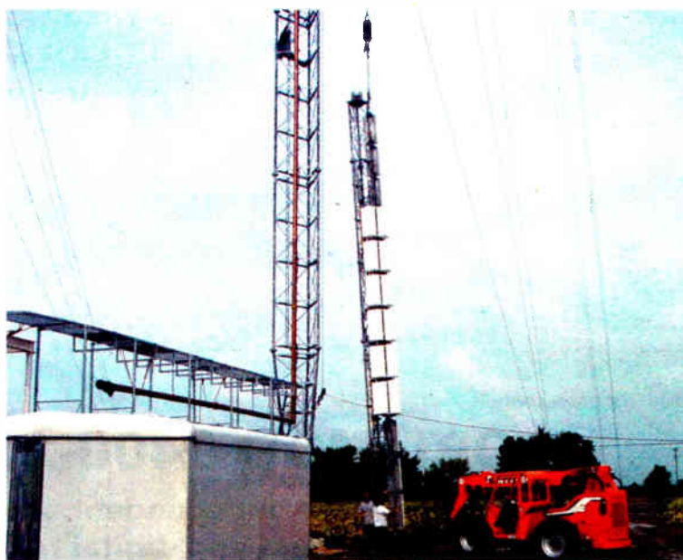
PSI installs a high-power broadband panel system for a Barrington Broadcasting Corp. television station in Bay City, Mich.
