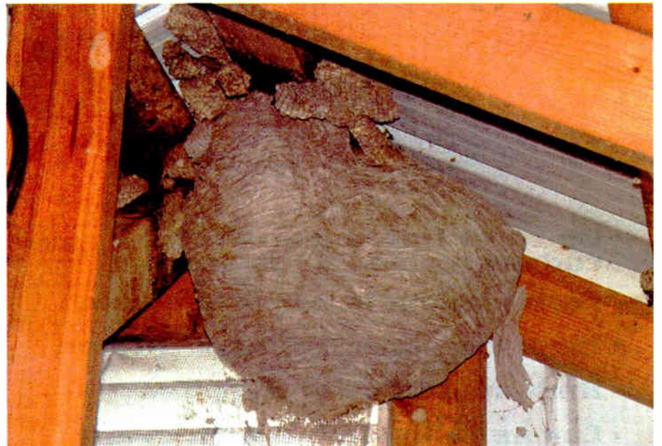
Fig. 3: Who knows what's lurking in your transmitter building attic?
