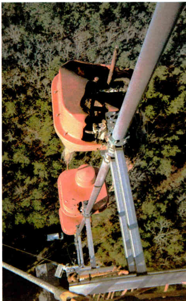
Fig. 2: Lightning melted this radome.
