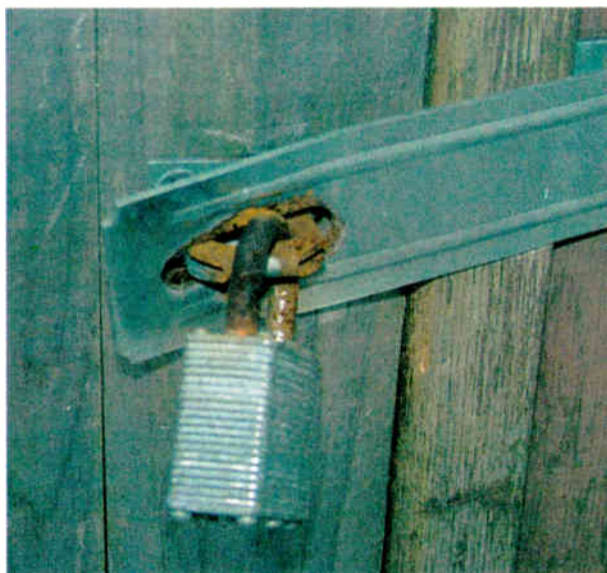
Fig. 2: Make a visual inspection of transmitter site locks and hasps at least once a year.
