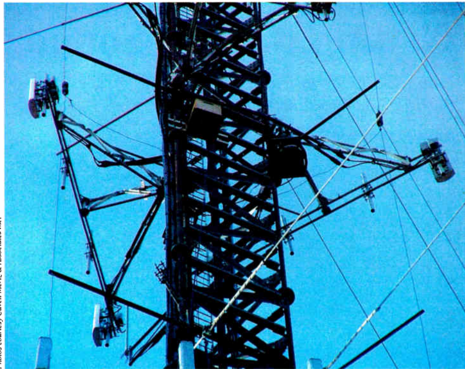
AM tower hosting wireless antennas.
