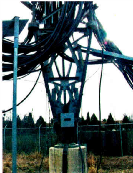
Busy grounded tower base
