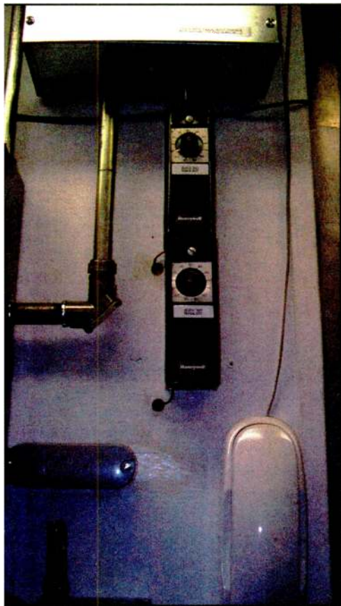
A consolidated control system with temperature controls and an off-the-shelf electrical enclosure for the relay and current sensor mounted on the electrical power wall. The sensing bulb is slightly larger than the capillary tube, so an oversized hole to clear the bulb was drilled for each sensor to pass these through the plywood wall and then onto the outside. Caulk was used to fill the excess space in the holes as well as to stabilize the position of the tubes.
