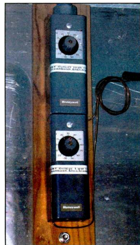
Interior mounted temperature sensor controls with high on top (set at 38° F) and low on bottom (set at 20° F). This station wanted absolutely no possibility of icing (a big biller) and so set a wide window. Since these two units create essentially a single-pole switch, only two wires are needed to interconnect with the main control assembly on the other side of the room near the electrical equipment.
