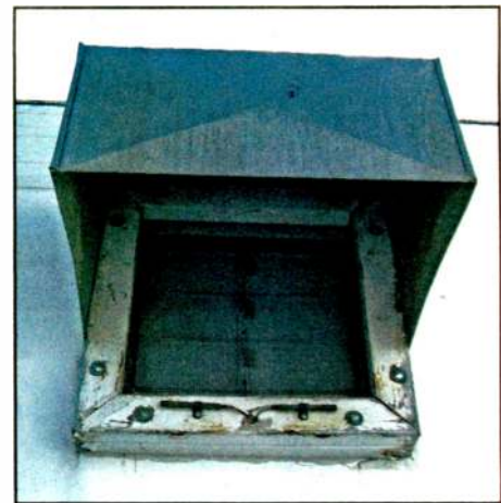
High and low remote temperature sensing bulbs mounted on the wooden frame of a fresh air input vent on the north side of the transmitter building. The wood conducts less of any ambient heat to the sensors and the shroud shields the sensors from rain and ice.
