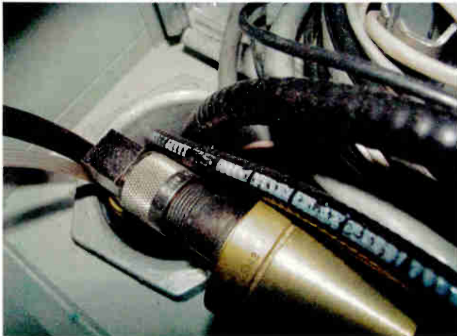
Fig. 1: Before sealing conduits, ensure they are water-free to avoid damage to cabling.
