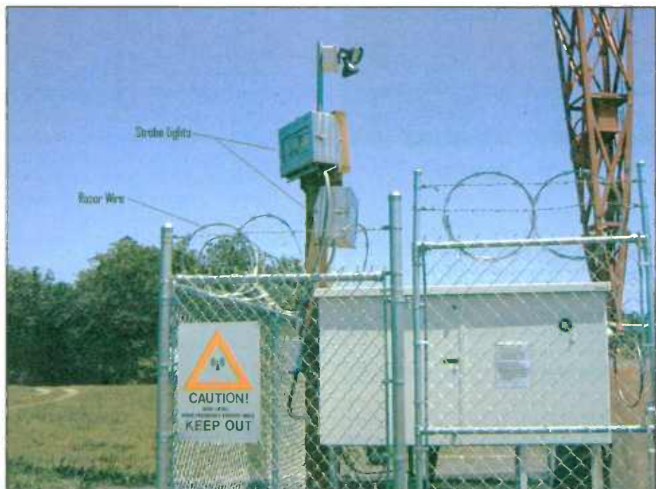
A real attention-getter: Tower strobes pulsing with several hundred thousand candelas when the tower base alarm trips. Razor wire discourages the over-the-top approach to tower base entry.
