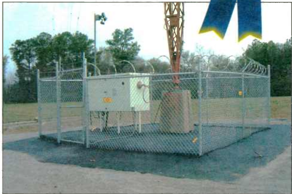
Blacktop was installed to cover the vulnerable ground screen and strap at each tower base.
