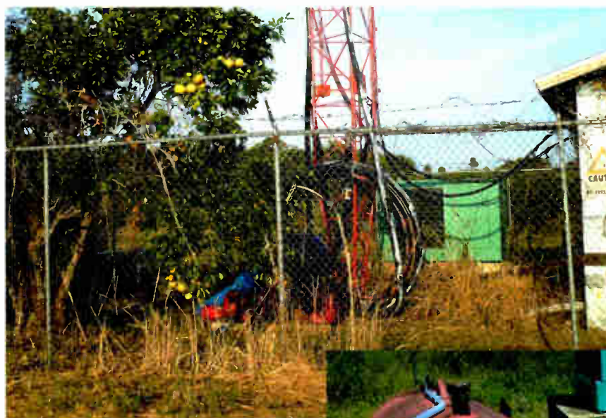
Fig. 1: Even a short coil of coax can tempt a thief.
