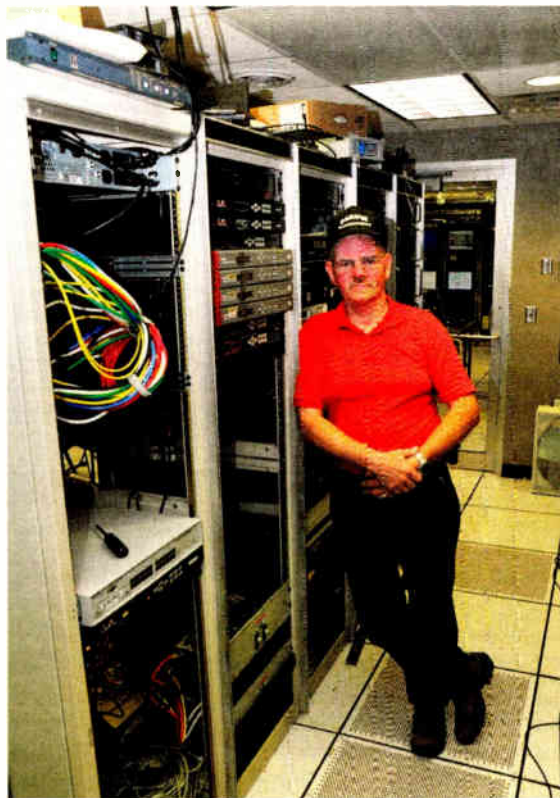
Don Forseth, technical services coordinator for South Dakota Public Broadcasting, stands in the server room of the Network Operations Center in Vermillion, S.D. He says the loss of PTFP funding means emergency grants used by public broadcasters when a major equipment failure hit in the past will not be available.
