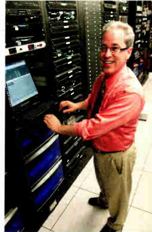
Wayne Gignac in the rack room.
