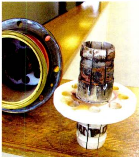
Fig. 5: The line bullet is heavily discolored, indicating overheating.
