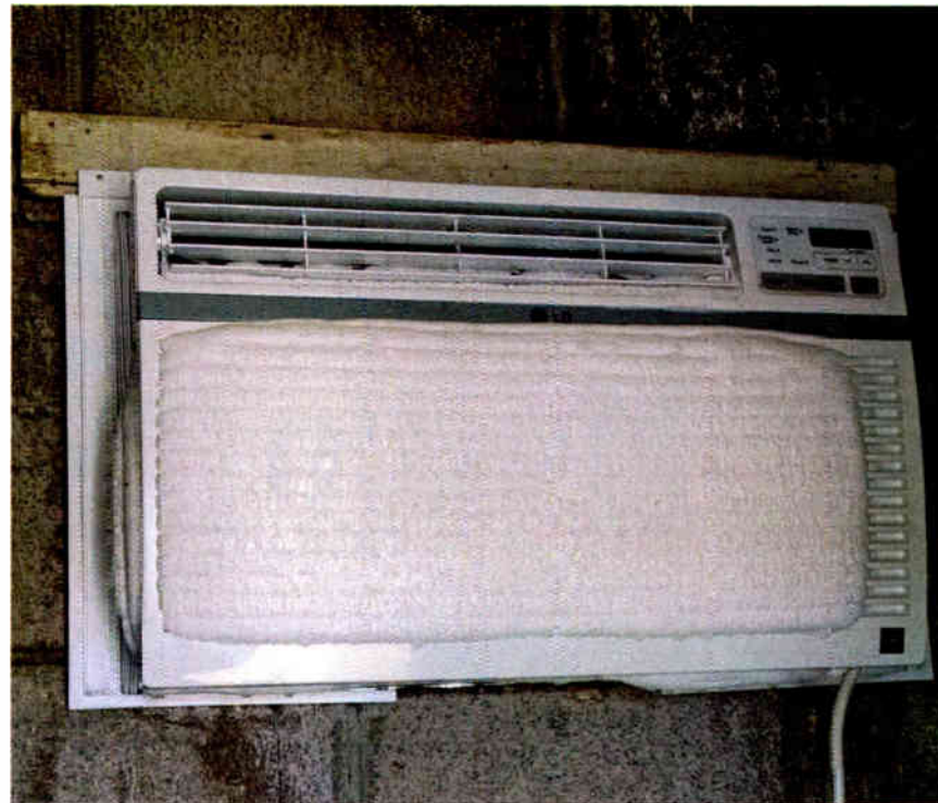
Fig. 1: A routine site inspection found this frozen air conditioner.
