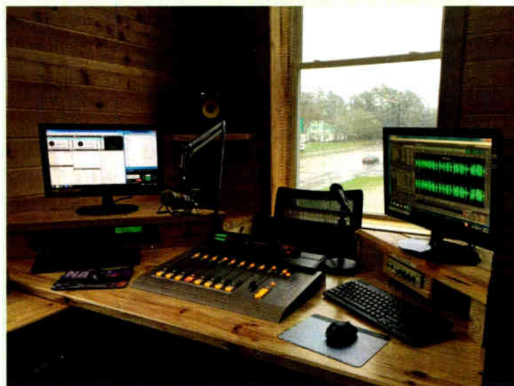
The control room of WBSC(LP), which was completed in April 2015. Hand crafted from cedar in a 19th century former hotel. Harris Oasis console ... and yes, you can play vinyl on the air.
