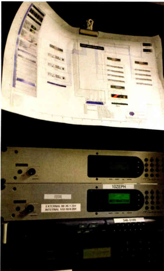
Fig. 1: Documentation drawings are placed above each rack.
