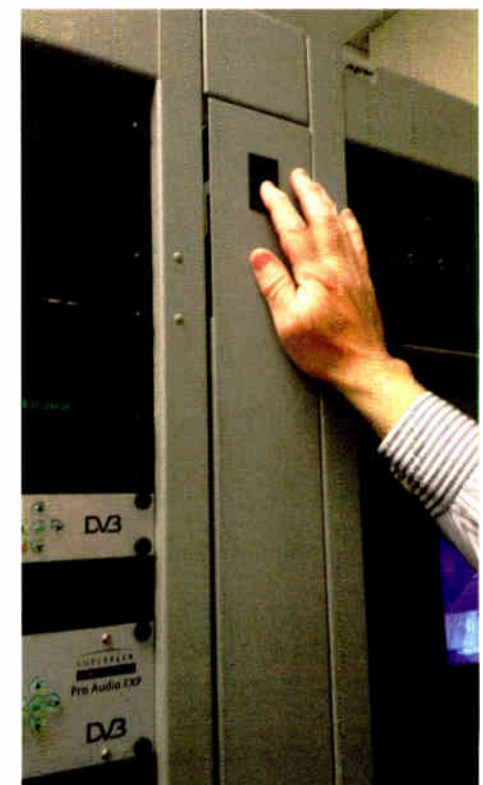
Fig. 2: The divider provides plenty of space to route cables.
