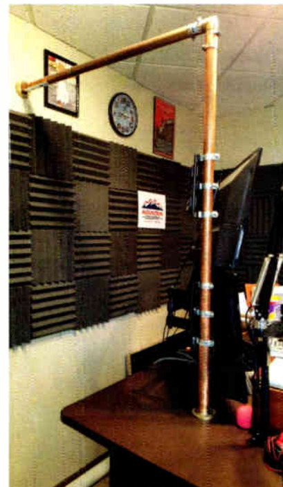
Fig. 2: The rigid line actually supports the control room monitors.
