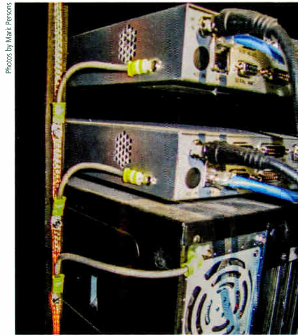
Fig. 3: Good grounding in a wooden rack.
