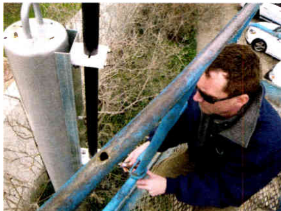
Information Station Specialists technician Geoff Penna installs a TIS radio antenna at a Customs & Border Protection port of entry along the U.S./ Mexican border.
